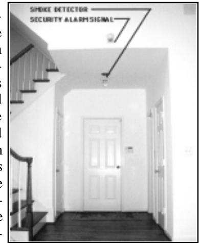
Photo of foyer -- shows the smoke detector and security alarm signal.
